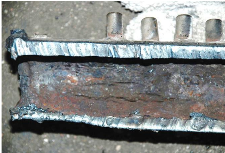
Photo 3: deposits around gouged section
